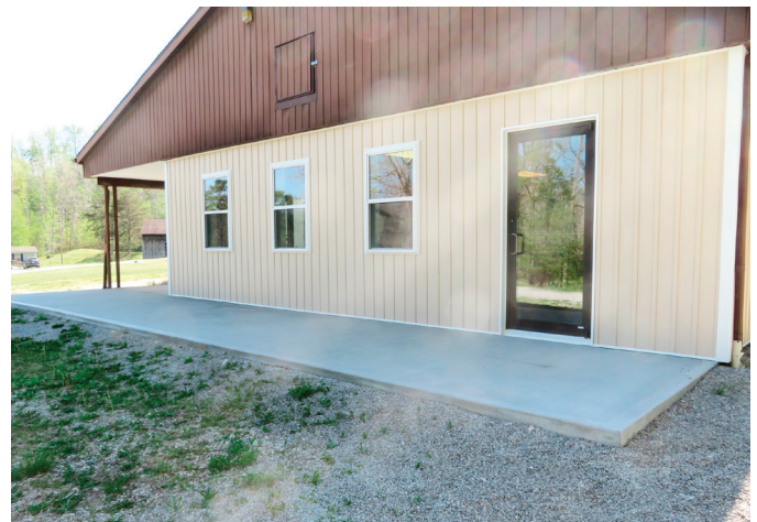
The porch expansion will provide more spaces for campers to gather outside. An additional door was added to the dining hall to provide easier access to the porch expansion.
