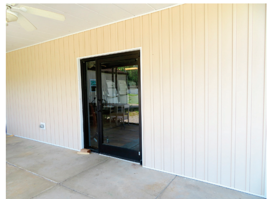
This exterior siding update helps ensure the stability of the building. Additional insulation was installed to help cool and heat the dining hall more efficiently.
