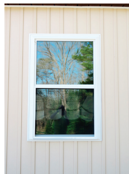
These new windows will improve energy efficiency, allow more sunlight into the dining hall, and will be easier for campers and counselors to open and close.
